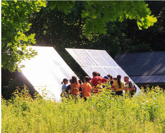
Ground mount solar at Mass Audubon's Pleasant Valley Wildlife Sanctuary in Lenox, Massachusetts.
