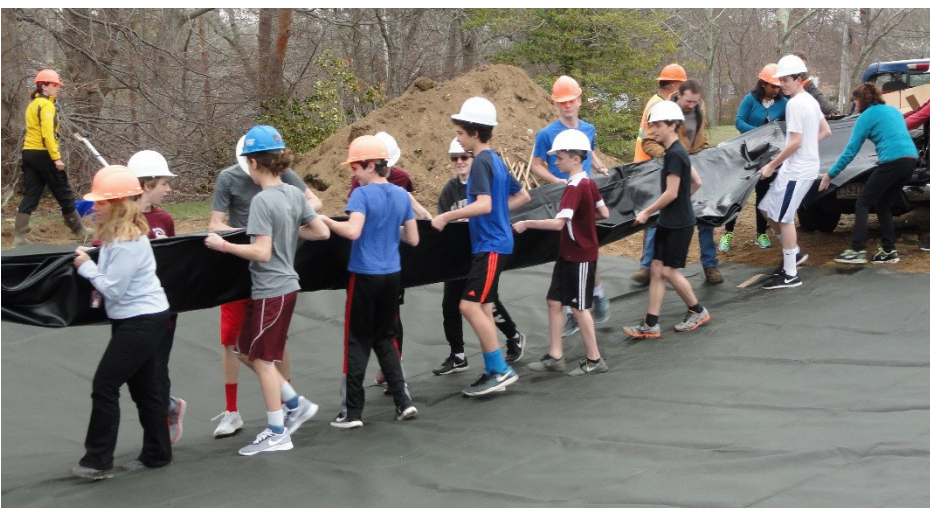
Seventh grade students at the Lawrence Middle School in Falmouth place the liner into the dug wetland depression.
