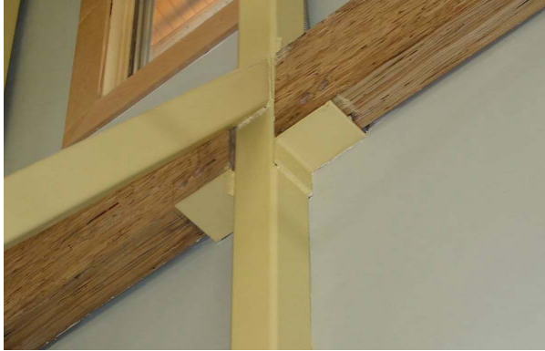
The building uses recycled steel and Parallel Strand Lumber (PSL) manufactured from wood fibers normally wasted in the milling process.
