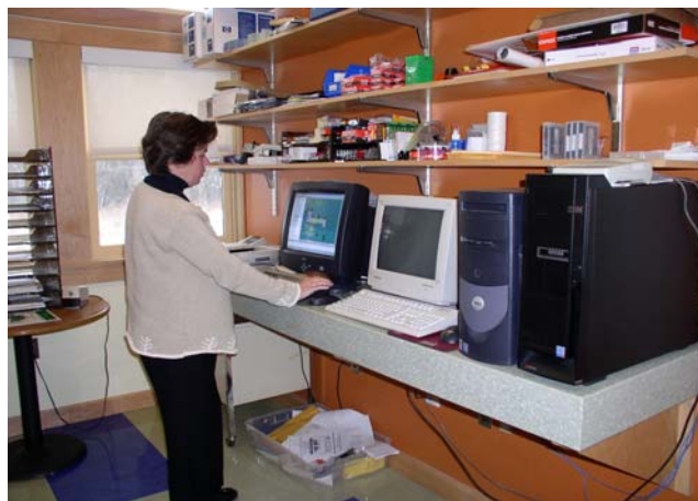
Sanctuary Director, Julie Branden, uses the workstation that controls the building's temperature and ventilation.
